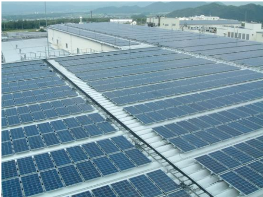
Solar Panels installed on the rooftop (Shiga Yohkaichi Plant)
